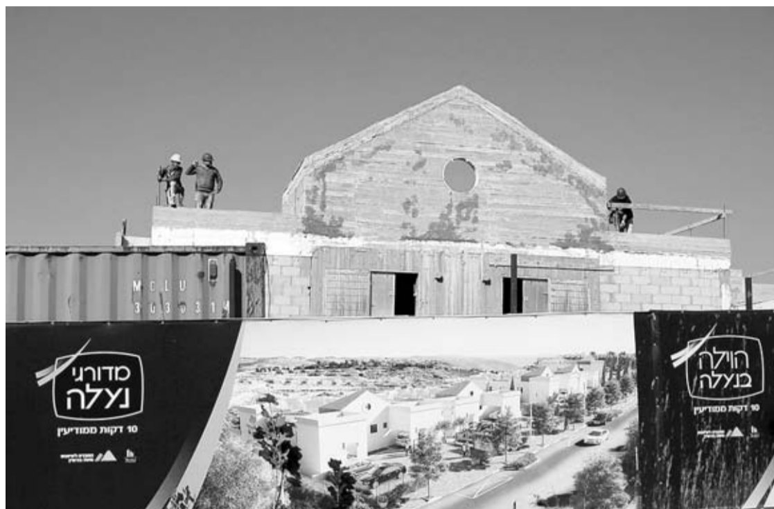
In this Tuesday, Jan. 1, 2019 photo, men work on a new housing project in the West Bank settlement of Naale.
